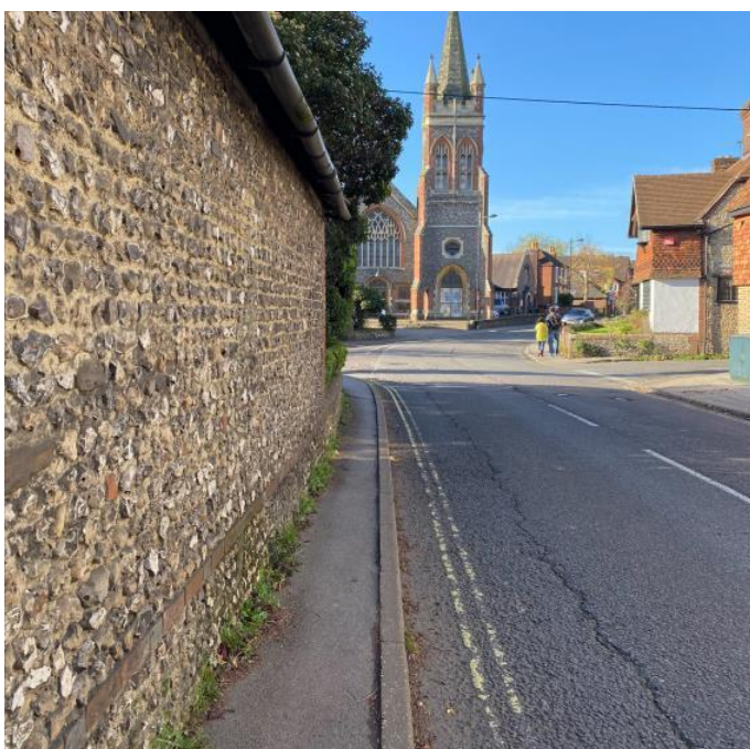
Figure 10: The extremely section of narrow pavement in Station Road, see WR3.4.3.
