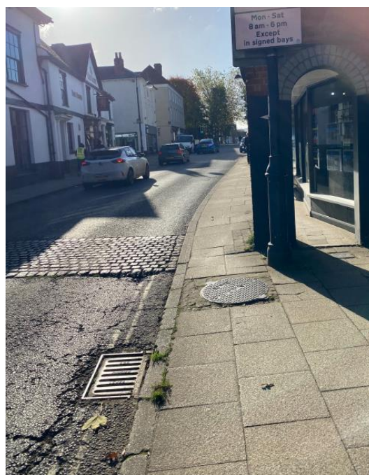
Figure 11: Damaged kerbs in Dragon Street, see WR3.5.3.
