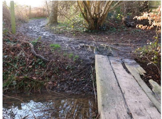
Figure 7: PROW 189/42/1 crosses a stream on a rotting bridge behind near No 6 Reed Way. Note the mud.
